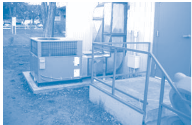
Figure 1 - Wall mounted heat pumps make classrooms too noisy for learning. This older bungalow classroom was affordably quieted by replacing a noisy wall-mounted HVAC with the quieter exterior unit shown here. The above-ceiling air distribution system (not shown) was also upgraded.
