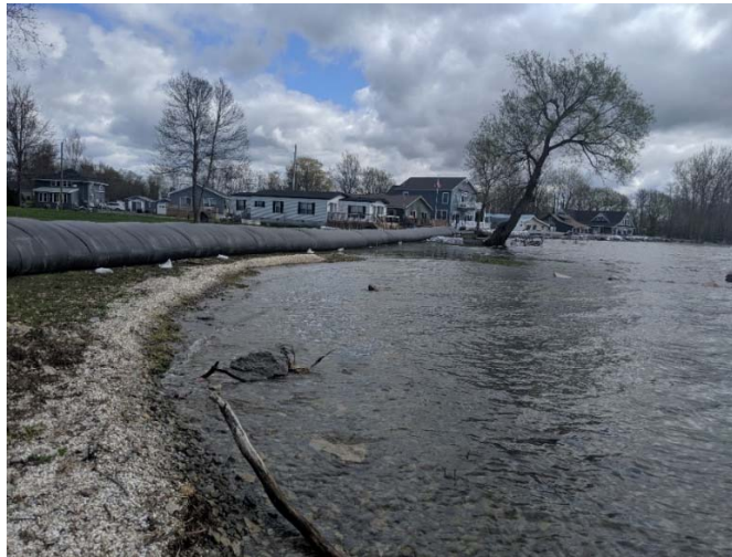
Figure 3.22 – Emergency response measures (e.g., Aquadam and supersack installation) may be warranted to protect properties that are not resilient
