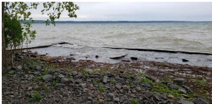
Figure 3.24 – A concrete seawall less than 50 years old becoming ineffective, due to changing conditions and limitations of material properties in design
